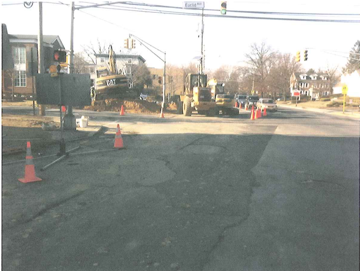
View of the Installation of the New Storm Sewer Inlets in Front of the TD Bank Property
