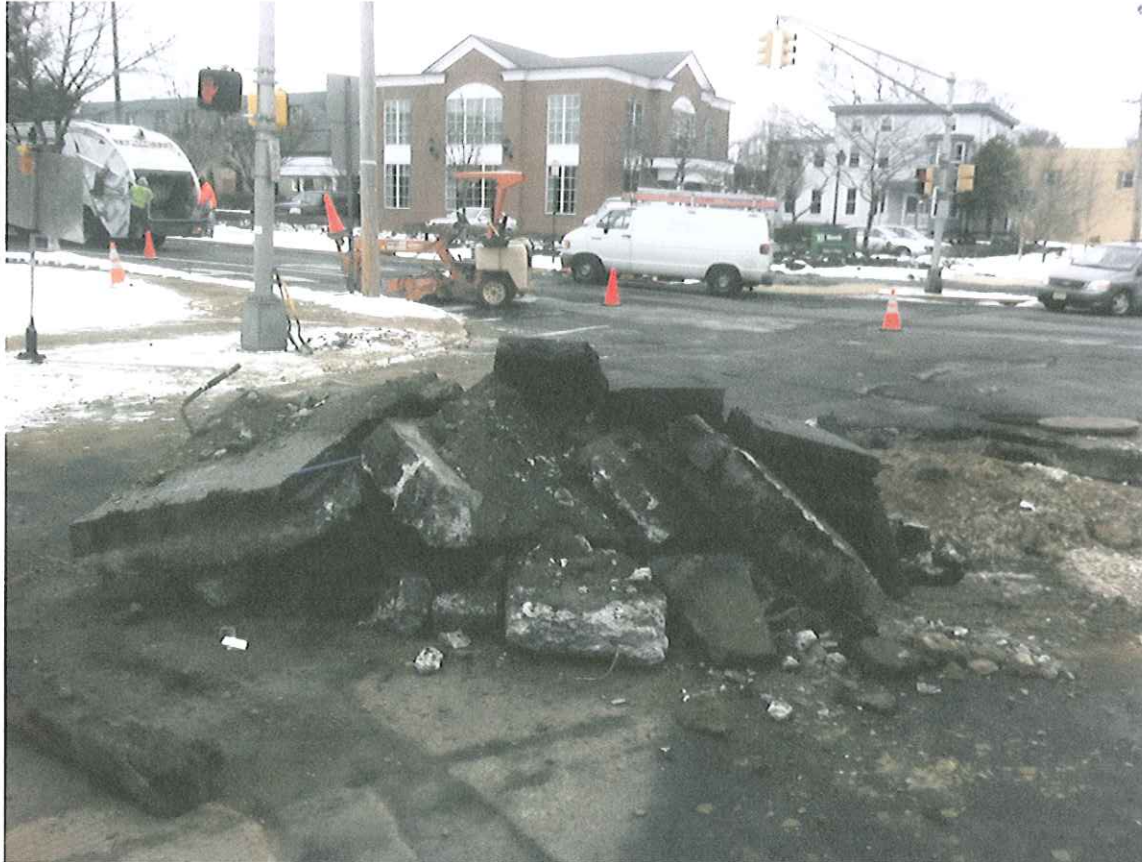
View of the Installation of the Final Sanitary Sewer Lateral for 89 North Haddon Avenue
