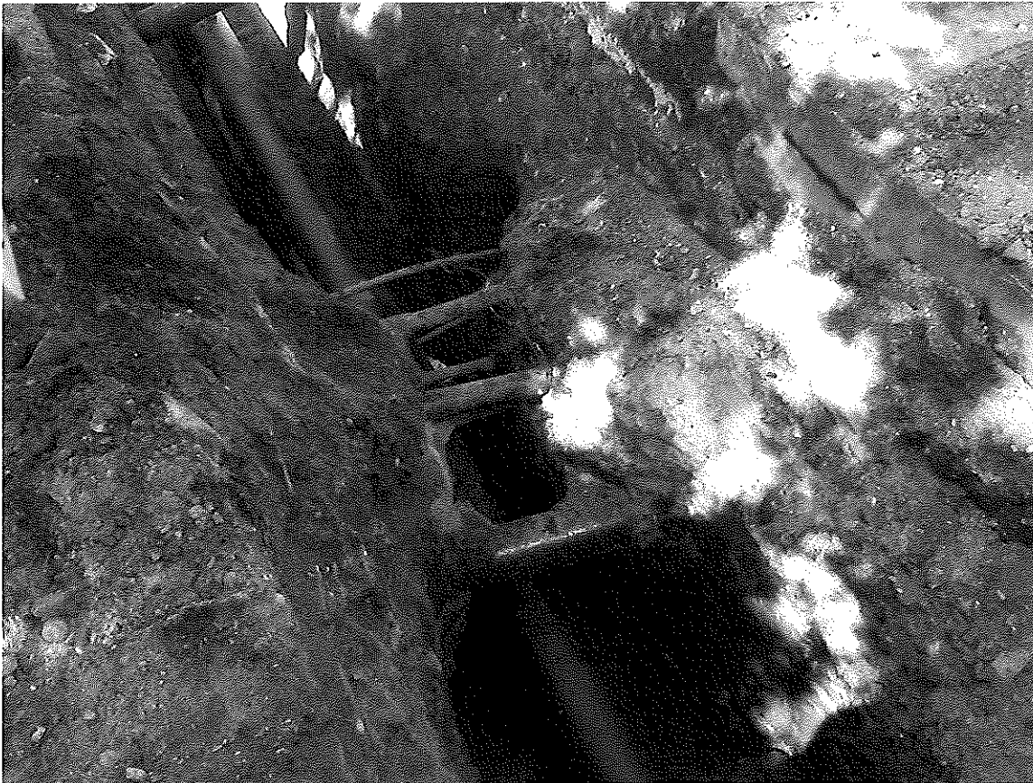
View of the Numerous Underground Utilities the Contractor Encountered During the Installation of the New Water Services Between Euclid Avenue and Stiles Avenue
