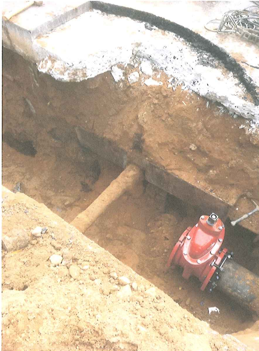
View of Existing Steel Sheeting Adjacent to the New 10 Inch Diameter Water Valve and Existing Gas Main
