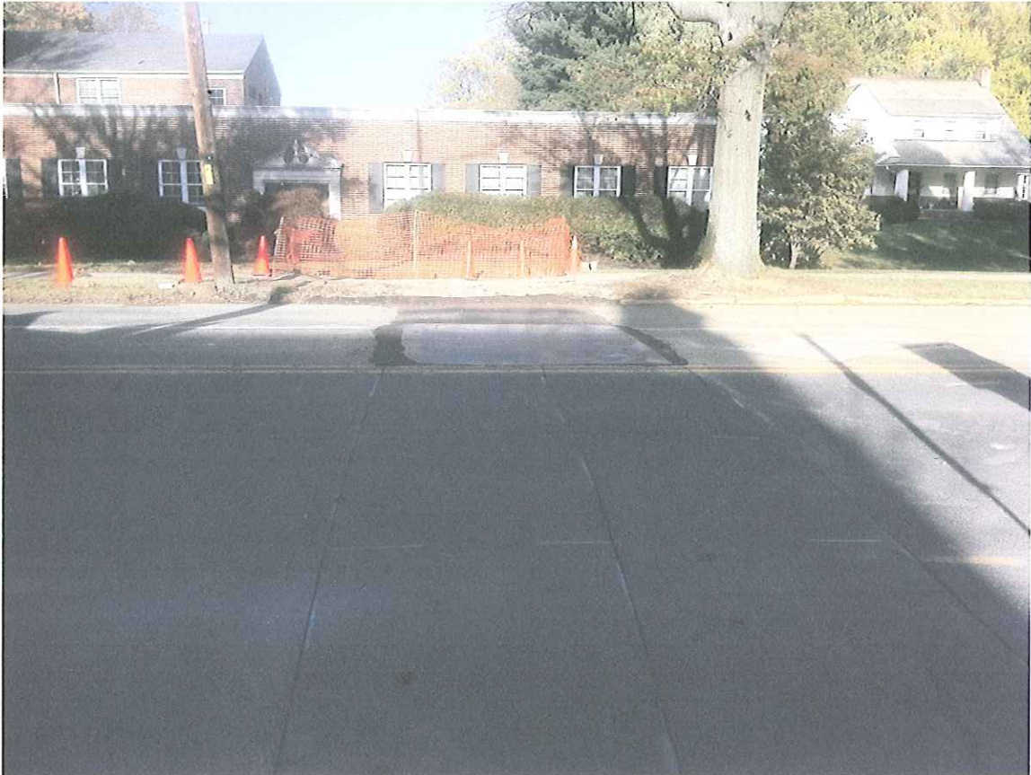
View of the Completed Storm Sewer Connection and Temporary Steel Plating on Haddon Avenue
