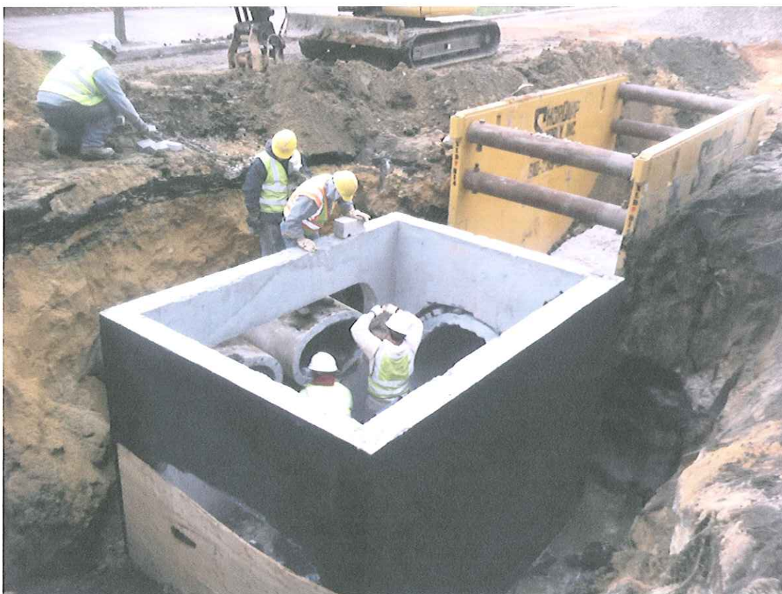
View of the Installation of the new 7-Foot by 10-Foot Storm Sewer Structure at the Library Point
