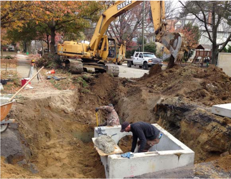
Installing New “Doghouse” Manhole at Estaugh Avenue Connecting New Stormwater System to the Existing System
