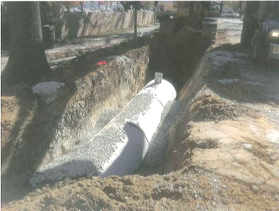
View of the Installation of the New Storm Sewer Piping along Tanner Street at the Rear of the 56 Haddon Avenue Property
