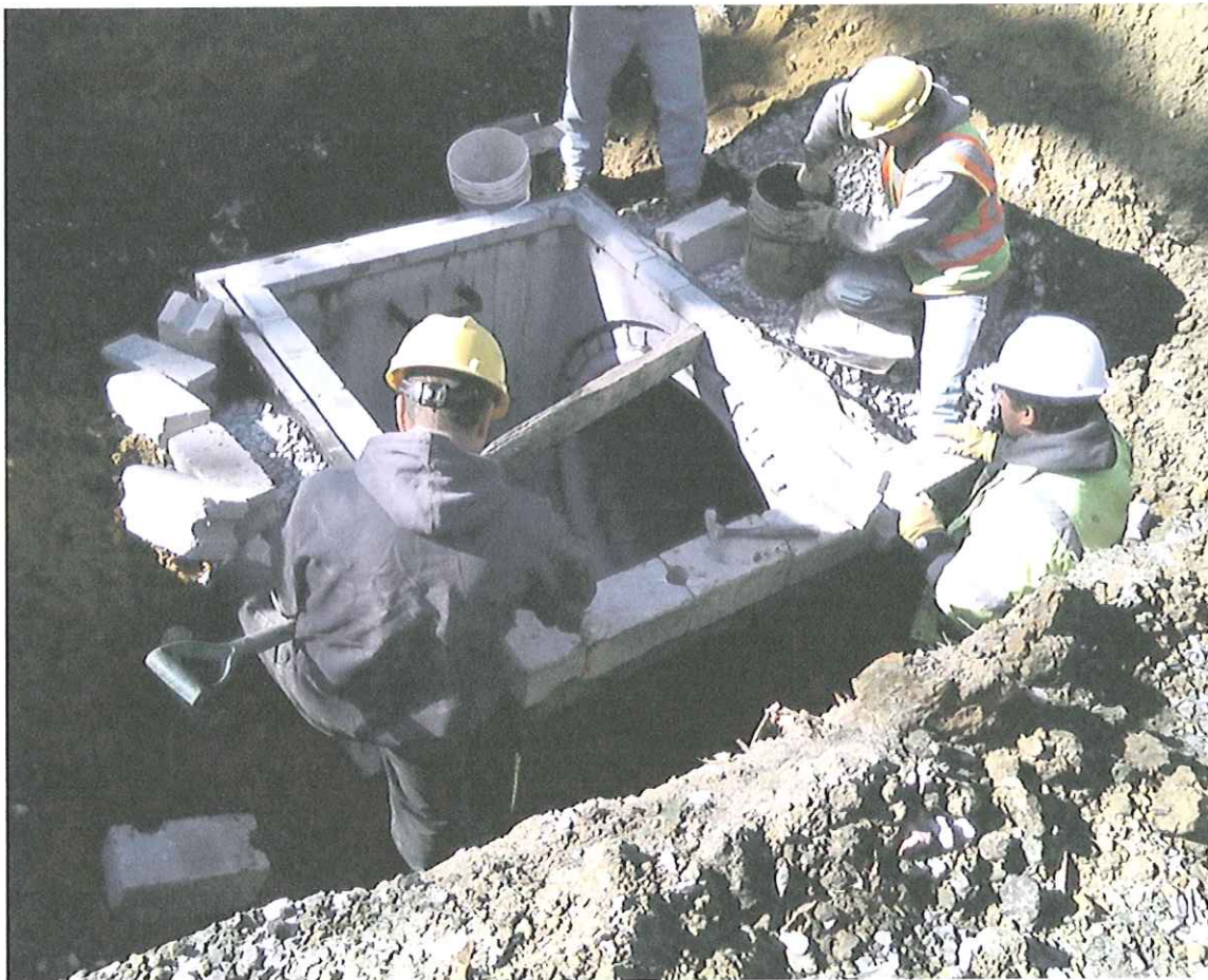
View of the Installation of a New Storm Sewer Inlet Structure at the Clement Street Intersection
