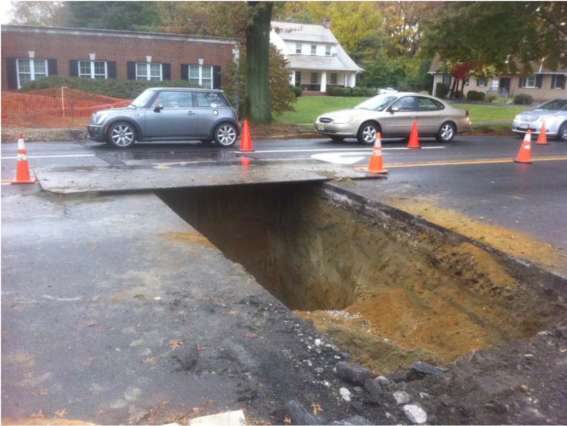
View of the Installation of the New 48 Inch Diameter Storm Sewer in Haddon Avenue
