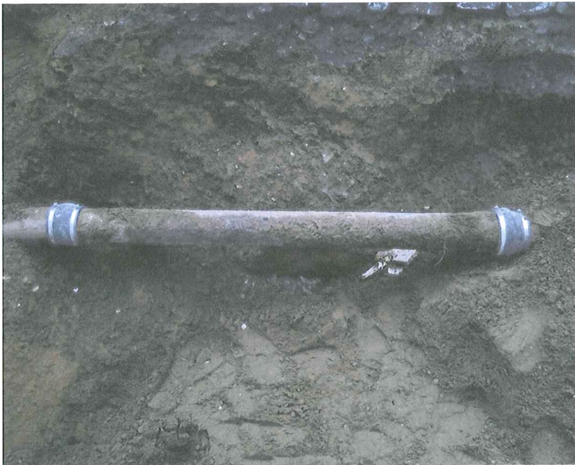
View of a Utility Repair on the Existing PSE&G Electrical Conduit at Clement Street
