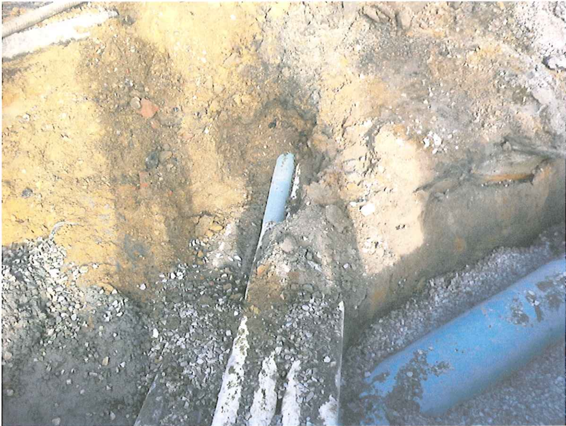
View of Some of the Existing Underground Utilities Encountered During the Installation of the New Sanitary Sewer Main at Euclid Avenue
