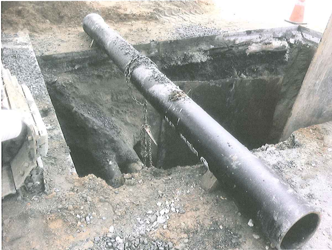
View of Temporary Support for Existing Underground Utilities Encountered During the Project
