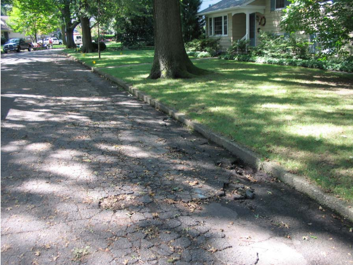
View of Existing Deteriorated Pavement along Pennbrook Drive
