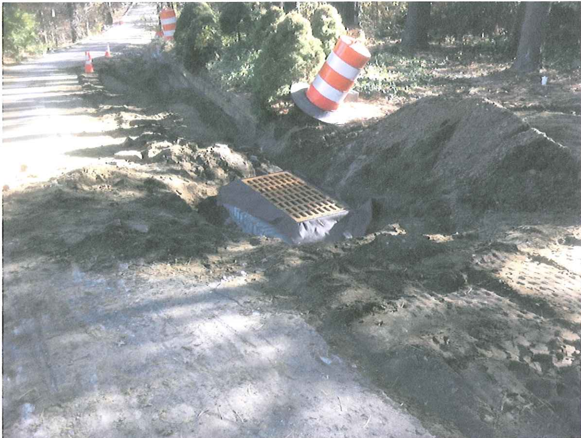
View of a Newly Installed Storm Water Inlet along the Private Driveway
