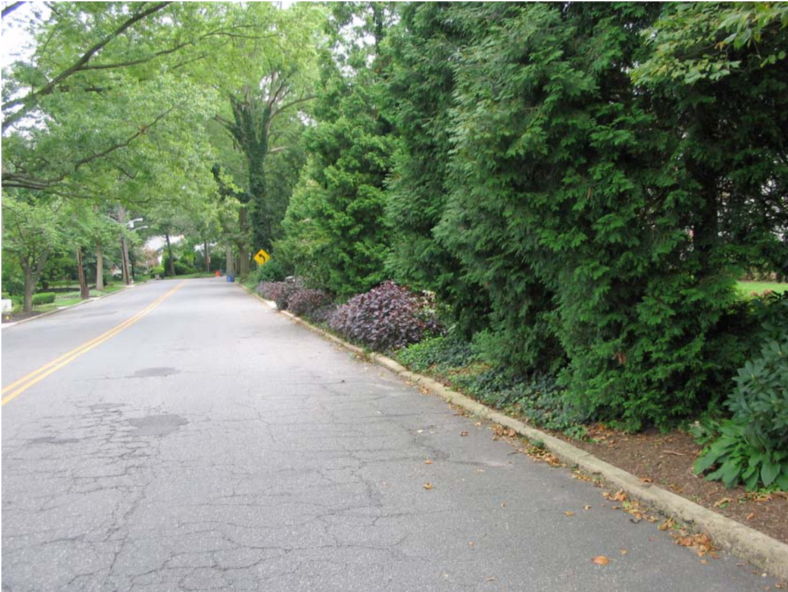
View of Existing Cracked Pavement along Station Avenue
