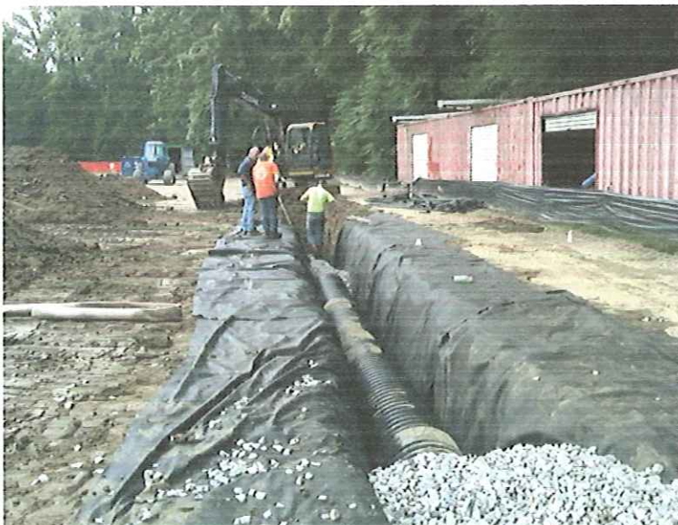
Installation of 24-inch Underdrain Pipe Along the North Side of Anniversary Field
