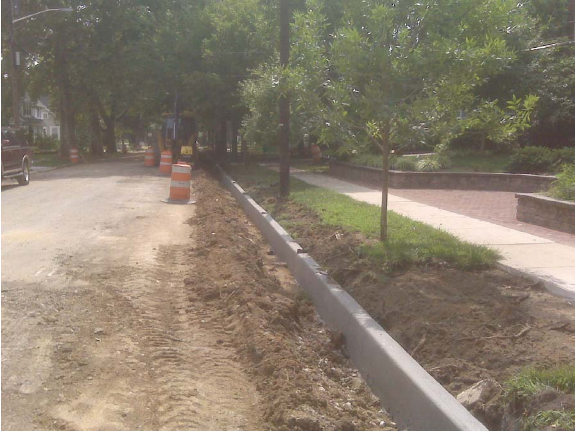
New Concrete Curb in Front of the Elizabeth Haddon Elementary School Property
