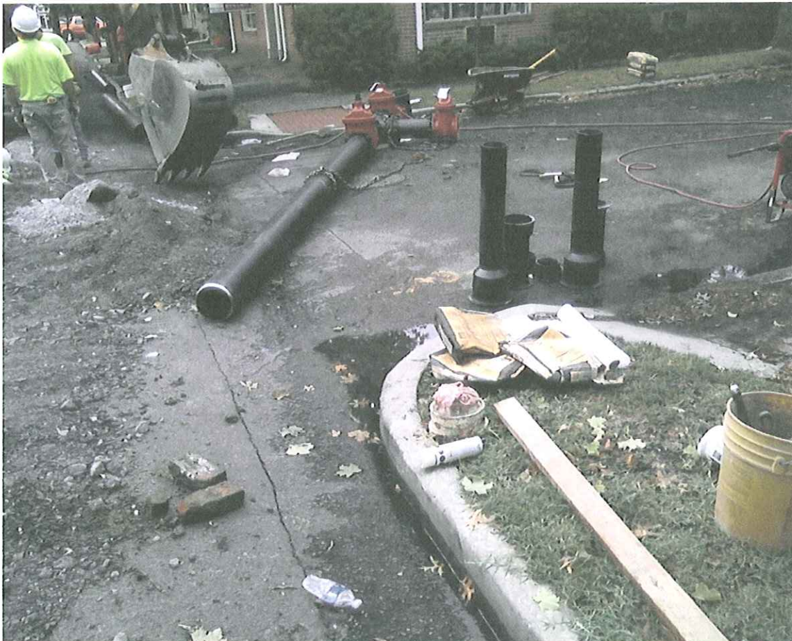
View of the New 8 Inch Diameter Ductile Iron Water Main and Valves Being Installed at the Intersection of Wilkins Avenue
