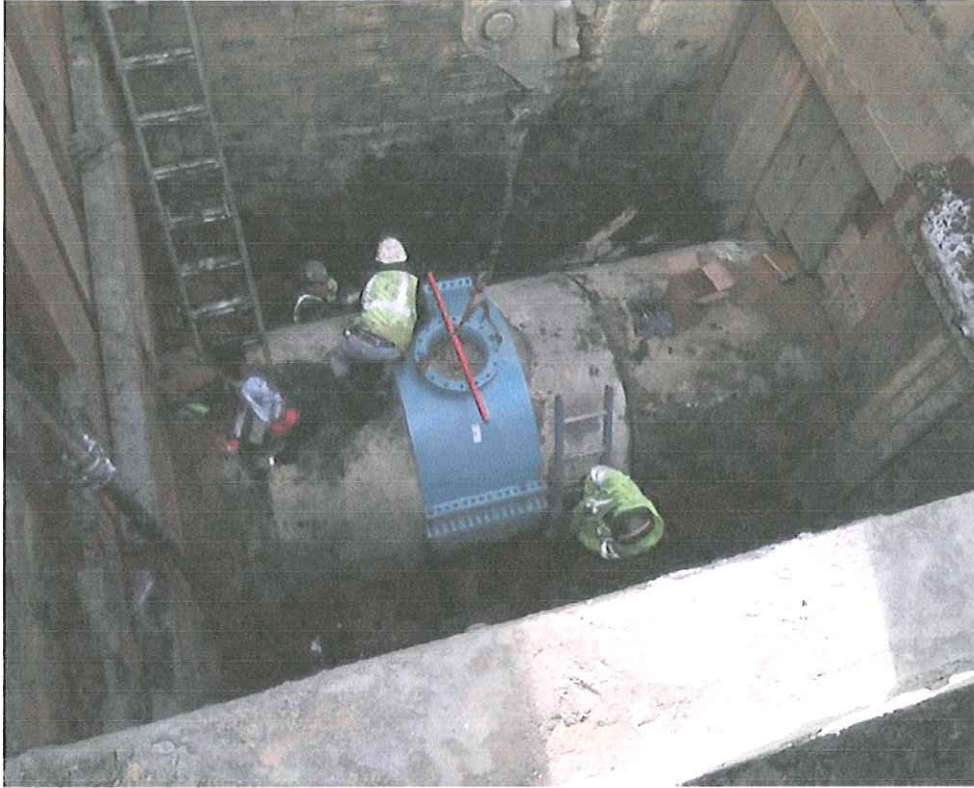
A tapping saddle (in blue) is installed around the interceptor pipe. The tapping saddle allows connection to be made to the pipe without interrupting the current sanitary flow in the pipe.
