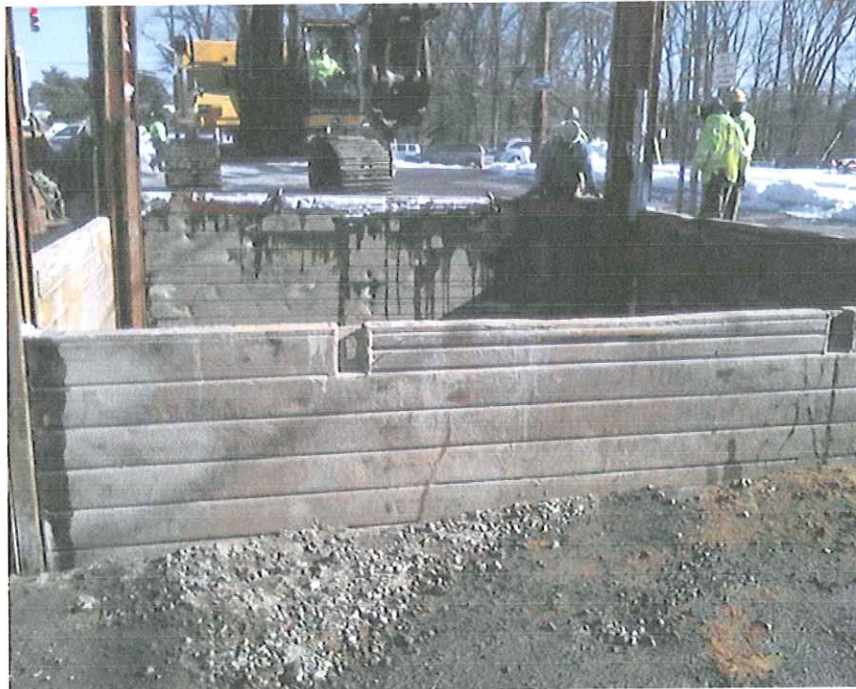
Due to the interceptor being 15 feet below the roadway surface, a trench box is being installed to prevent the walls of excavation from collapsing.
