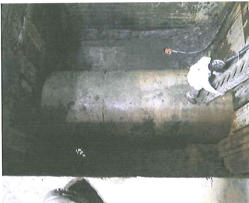
The top of the interceptor is exposed and workers begin preparing for the next step in making the connection.
