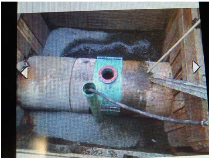
The saddle is completed so a connection can be made to the 66" CCMUA Interceptor. New gravity sanitary sewer will be attached to the interceptor.
