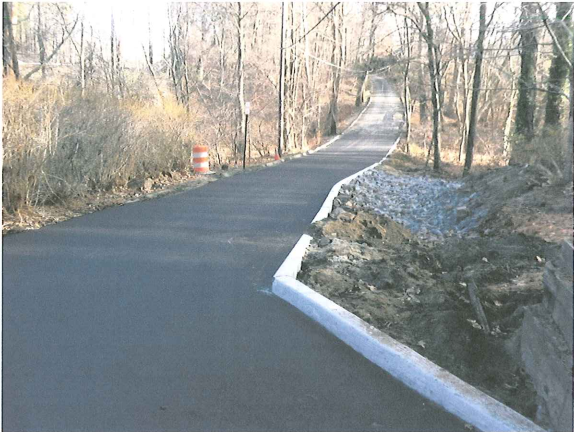
View of the Driveway at the Repaired Storm Water Outfall Location after the Paving Process Was Completed
