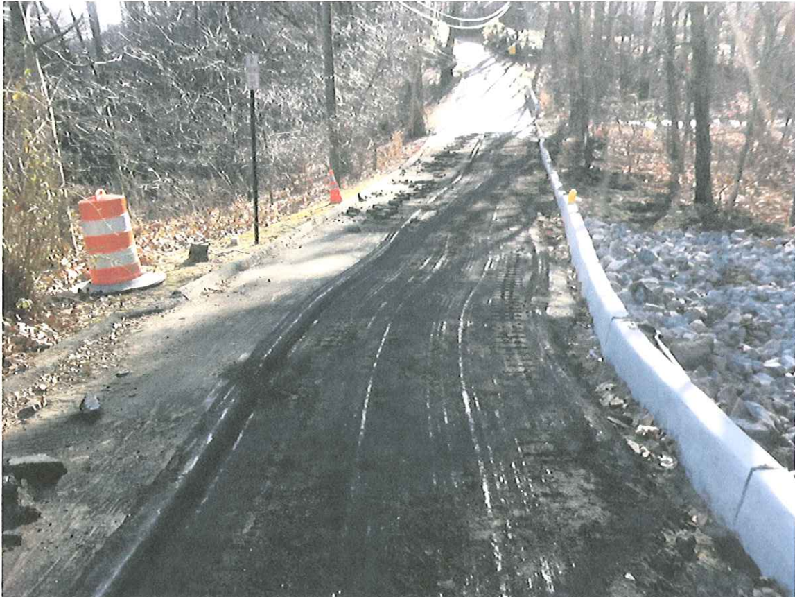
View of the Driveway at the Repaired Storm Water Outfall Location during the Paving Process
