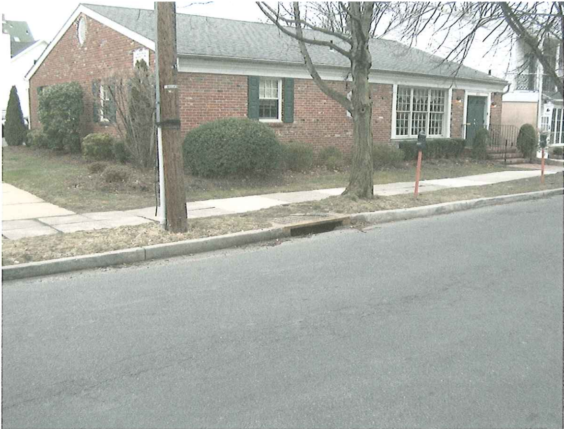
View of Existing Storm Sewer Inlet Near the Intersection with Wilkins Avenue
