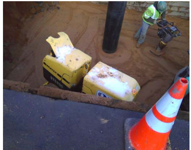
Workers compacted the backfill material over the newly installed gravity sanitary sewer. Proper compaction will reduce settlement and provide support to the existing and newly installed sanitary pipe.
