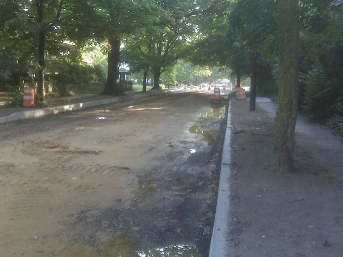
Wet Conditions on the 400 Block
